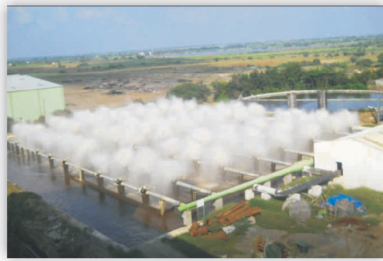
Advance Mist Cooling System.
